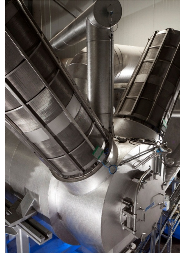
▲ Biomass torrefaction pilot plant in Frohnleiten, Austria. The energy content of torrefied biomass is 20% higher than that of white wood pellets.
